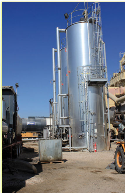
Figure 20. Auxiliary storage tanks
